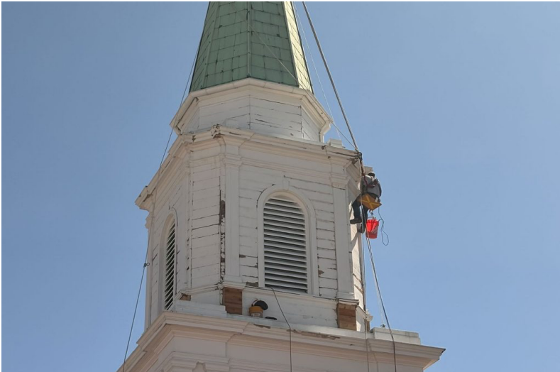
Aspire Church San Marco’s steeple underwent a restoration addressing leaks and other issues
